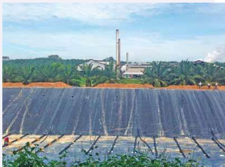
Biogas plant, Telok Sengat Mill
